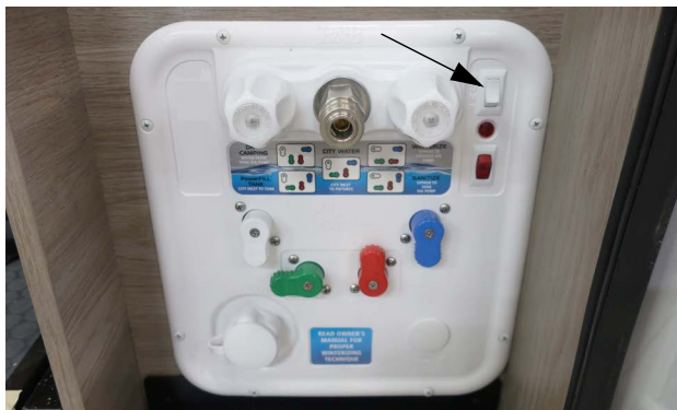
Pump switch -Typical View
