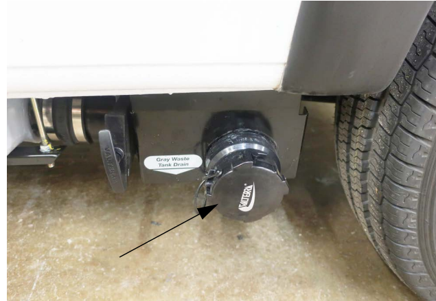
Sewage Drain Outlet (Located beneath motorhome on the left side) - Typical View
