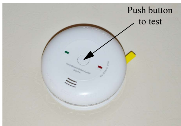
Carbon Monoxide Alarm
