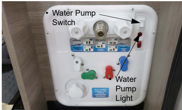
Water Pump switch located on Water Center Panel -Typical View
