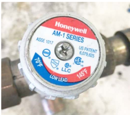
Hydronic Heating System Tempering Valve (Located below dinette seat - remove screws and panel to access)
