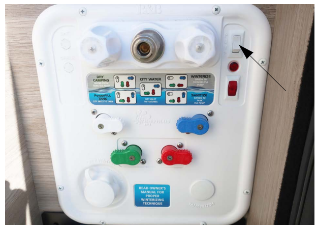
Water pump switch location on Water Center Panel -Typical View
